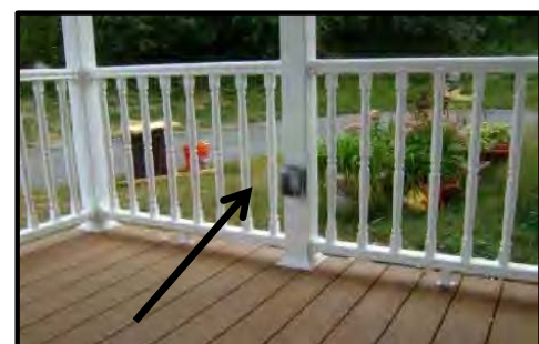
Electrical outlet inserted Into hollow post
